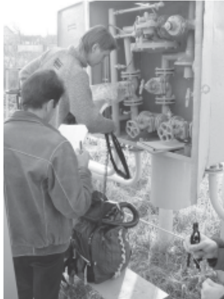
Maxim Alexandrovich with GasEnergy Technolog Ltd. measures a leaking valve at a regulator station in Kursk, Russia.
