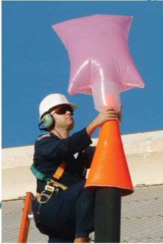
Unit Valve / Blow Down Valve Leakage
